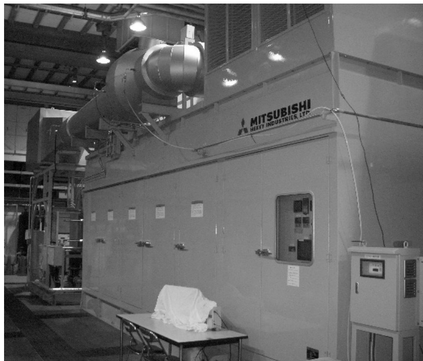
Fig.7 Picture of developed cogeneration package
